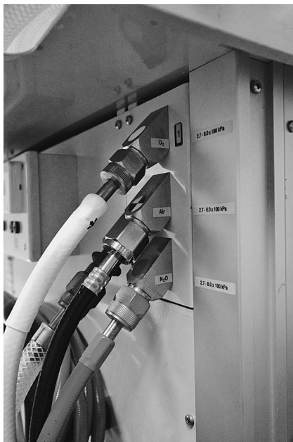
Fig 1.1 This image illustrates the pipeline connections at the back of an anaesthetic machine. Note the three hoses are colour-coded: oxygen is white, air is black, and nitrous oxide is blue. The pipelines are coupled to the machine at an NIST connector.
